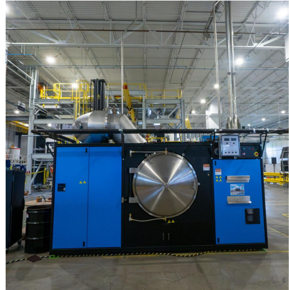
New sintering furnace delivered and being commissioned
